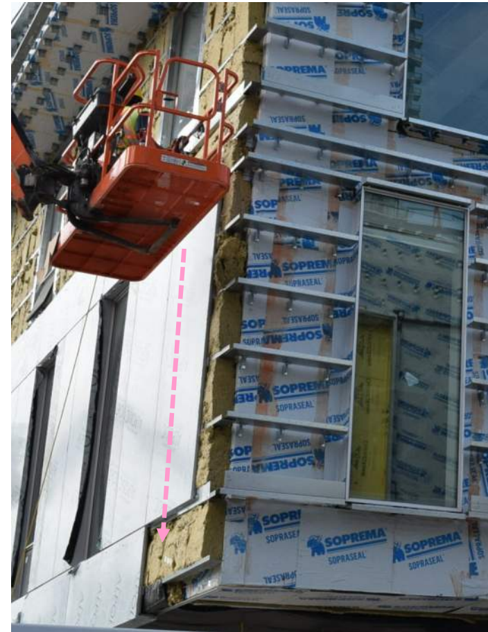
Airflow and drainage exterior of insulation in cladding profile, +shims at horizontals
