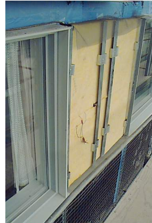
Bad thermally too - continuous Z-girts
