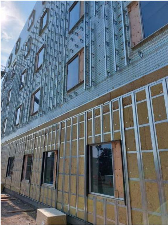
Steel hat framing - on thermal cladding attachment clips through exterior insulation over self adhered membrane WRB
